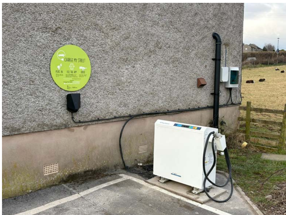
Recently installed and trialed V2X chargepoint at Yealand Village Hall
